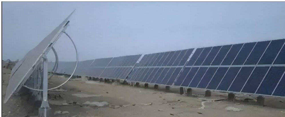
Figure 2. Tilt angle Adjustment for More power generation
