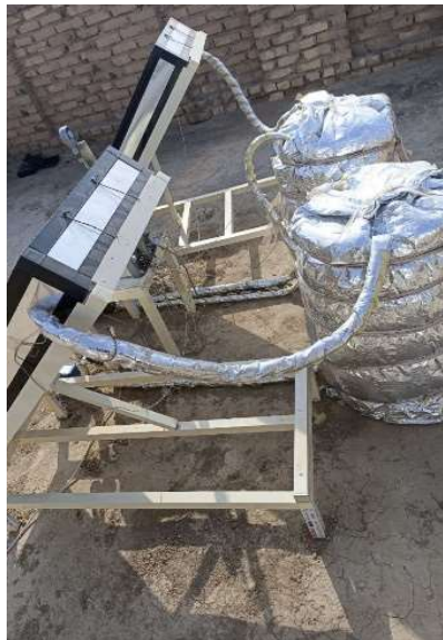
Fig. 6 Plastic pipes (1/2 inch) covered by insulators
