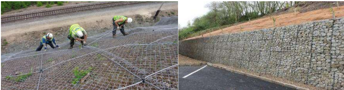
Figure 1. Protective device against falling stones and mountain avalanches in the railway.
