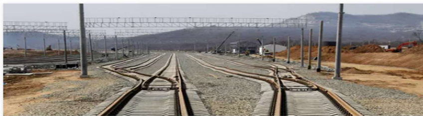
Figure 6. Aftermath of a landslide to the railroad.
